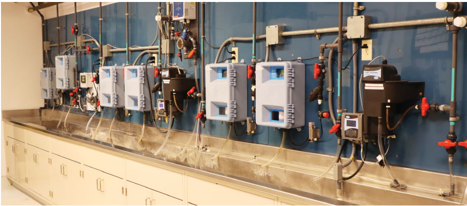
Water treatment at the Maplewood wellfield located at Maplewood Golf Course.
